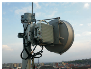
(1+1) system outdoor units directly mounted on a hybrid+antenna system
